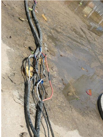
Figure 4: Frayed wires and power cables pose a significant electrical hazard. Image courtesy of marblegravy, Flickr.
